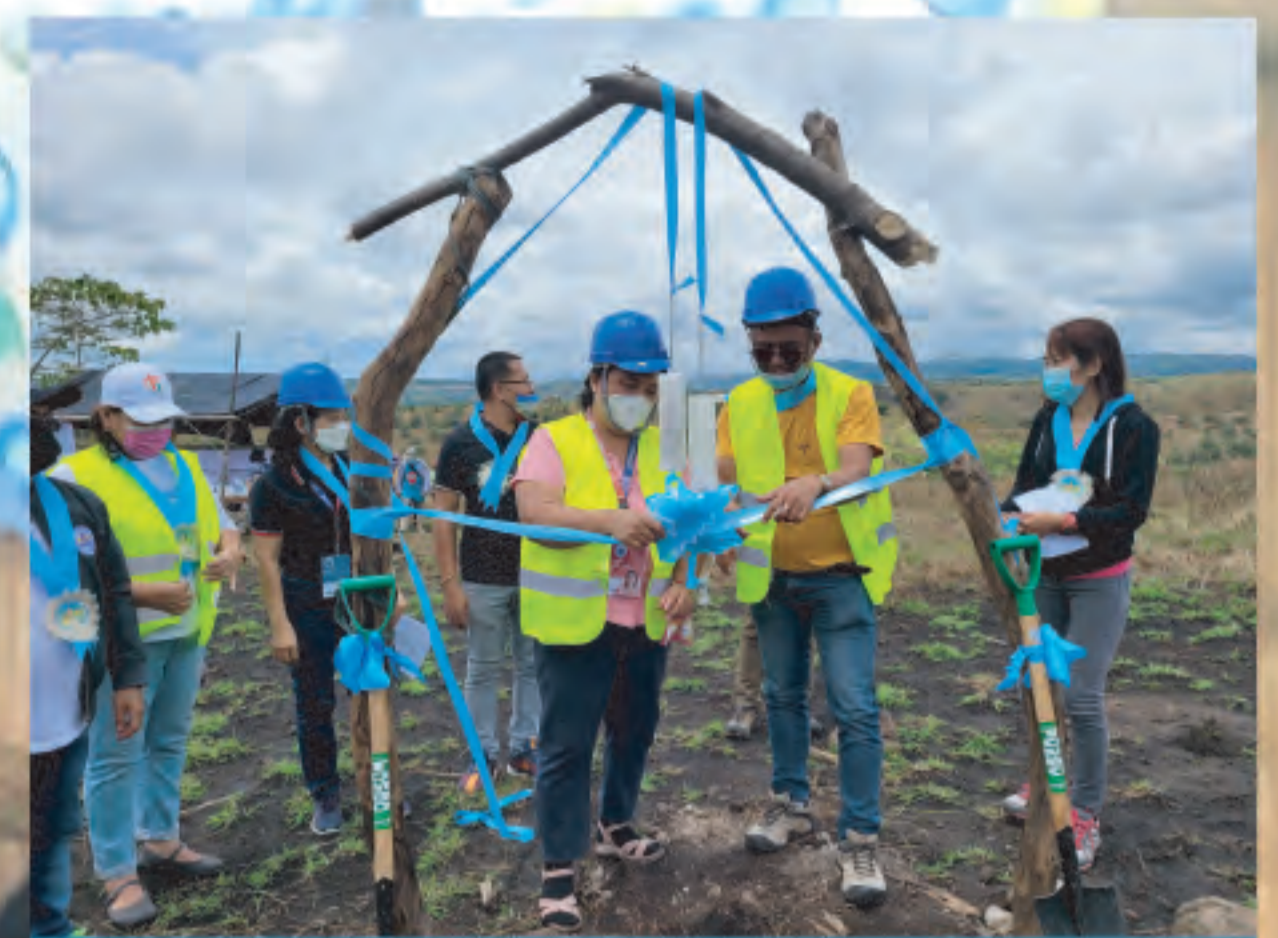
All hands on deck for the groundbreaking of Calfungal Elementary School which spurred excitement from the school's staff and community.
